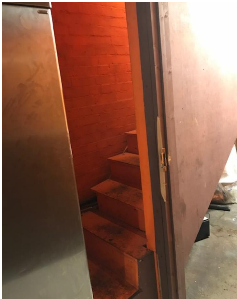
sf031 - Basement Area – Fridge blocking stairs Photograph taken on 13 June 2019 @ 12.14hrs
