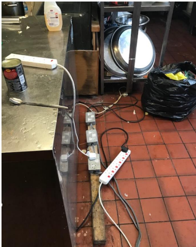
sf047 - Kitchen – Extensions leads and wires Photograph taken on 13 June 2019 @ 12.15hrs
