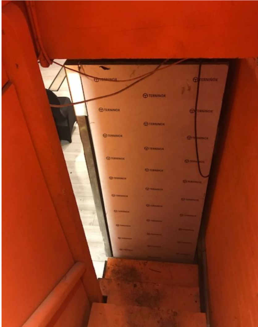
sf032 - Basement Area – Fridge blocking stairs Photograph taken on 13 June 2019 @ 12.14hrs
