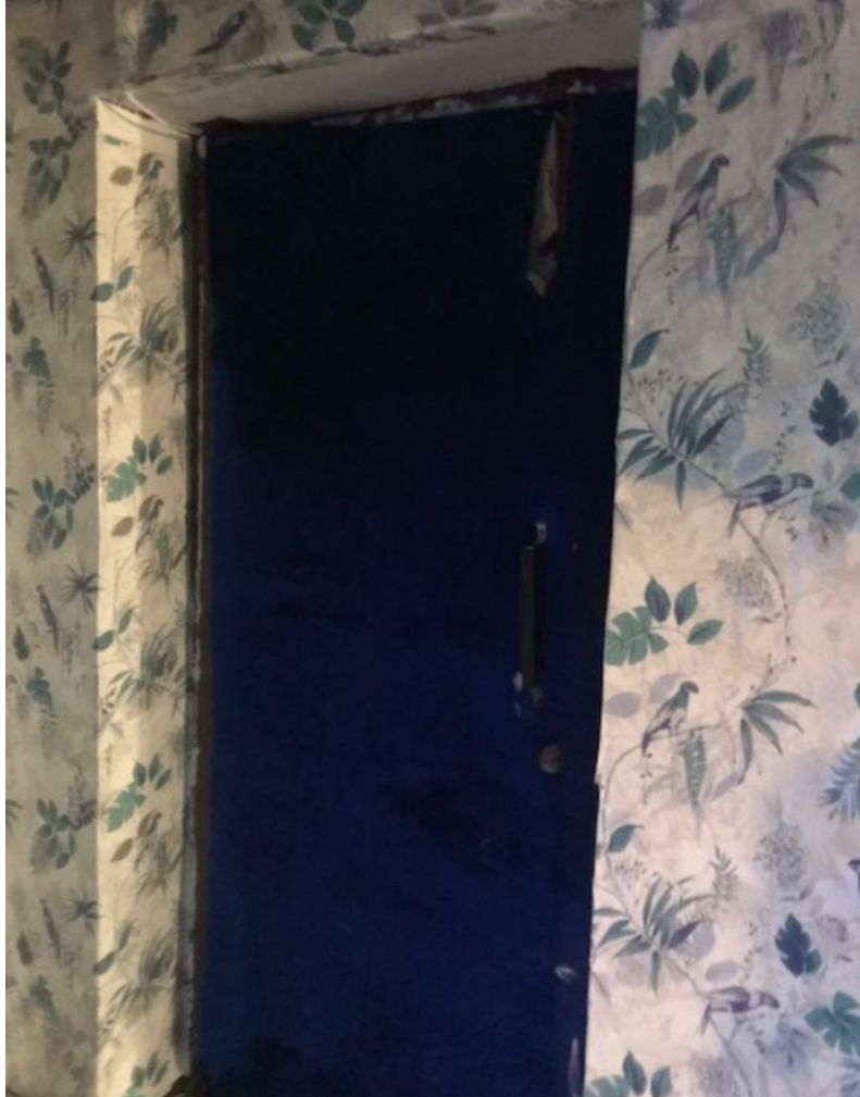
sf058 - Basement Area – Bolts on Fire Exit Photograph taken on 13 June 2019 @ 12.50hrs
