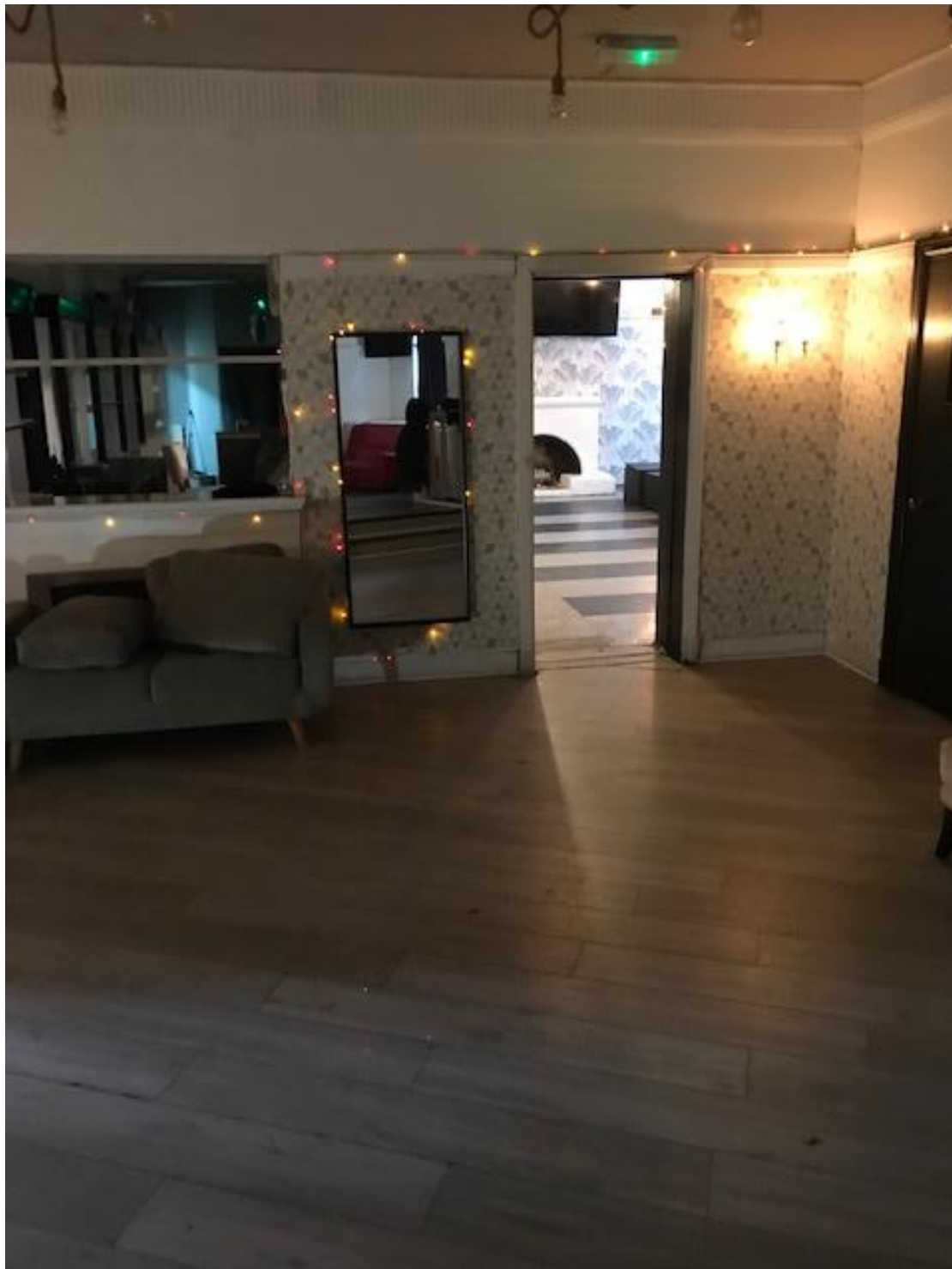
Ground Floor Customer Lounge – Water leakage from ceiling Photo taken on Thursday 13 June 2019 at 12:51hrs
