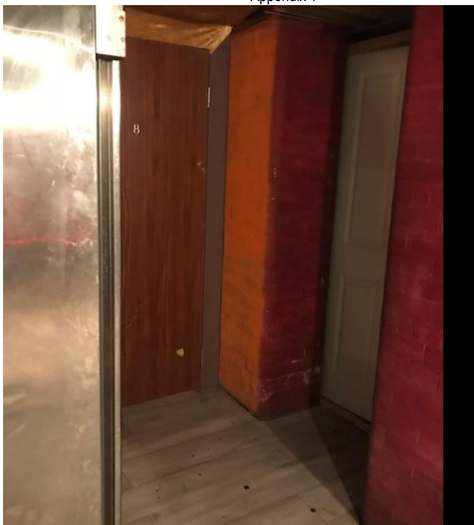
sf033 - Bedroom in Basement – Entrance to bedroom Photograph taken on 13 June 2019 @ 12.05hrs
