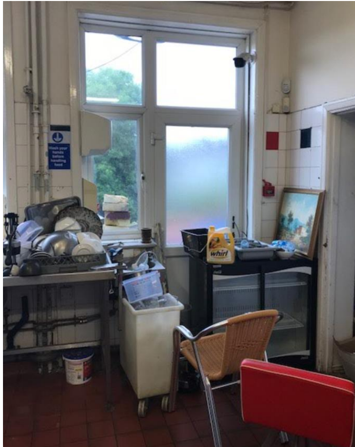
sf057 - Kitchen – Fire exit blocked internally and externally Photograph taken on 13 June 2019 @ 12.47hrs
